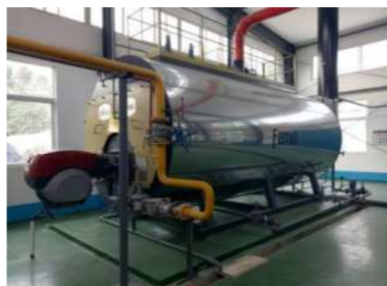
Natural gas boiler equipment ▶
