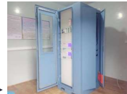
Online monitoring equipment ▶
